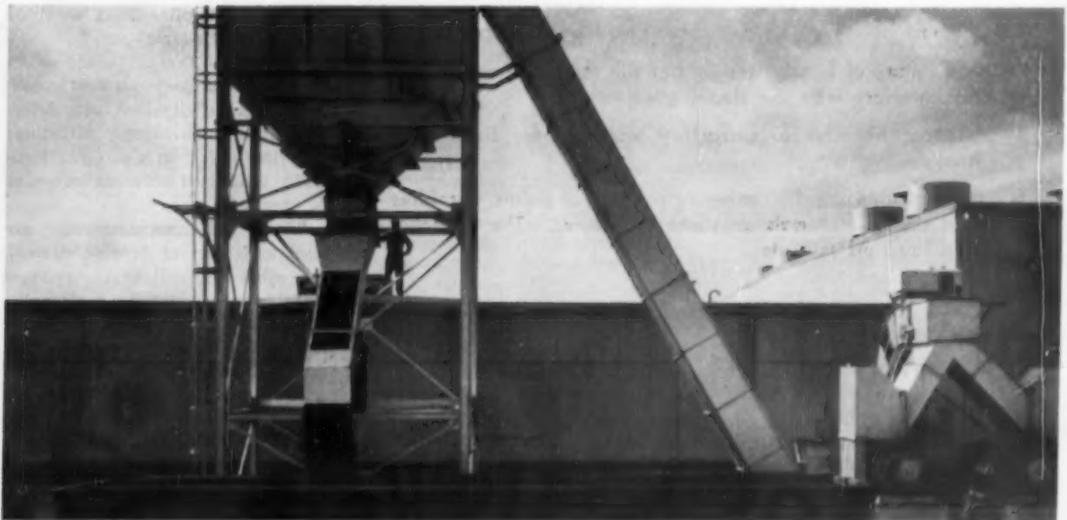
Both rough and finish machining departments are served by May-Fran chip removal systems. Chips fall from the machines onto conveyors, are moved along the lines and out of the plant. This hopper services rough machining; it has a double crusher to handle chips. Forty-two lb of steel is taken off each shell in rough machining alone
